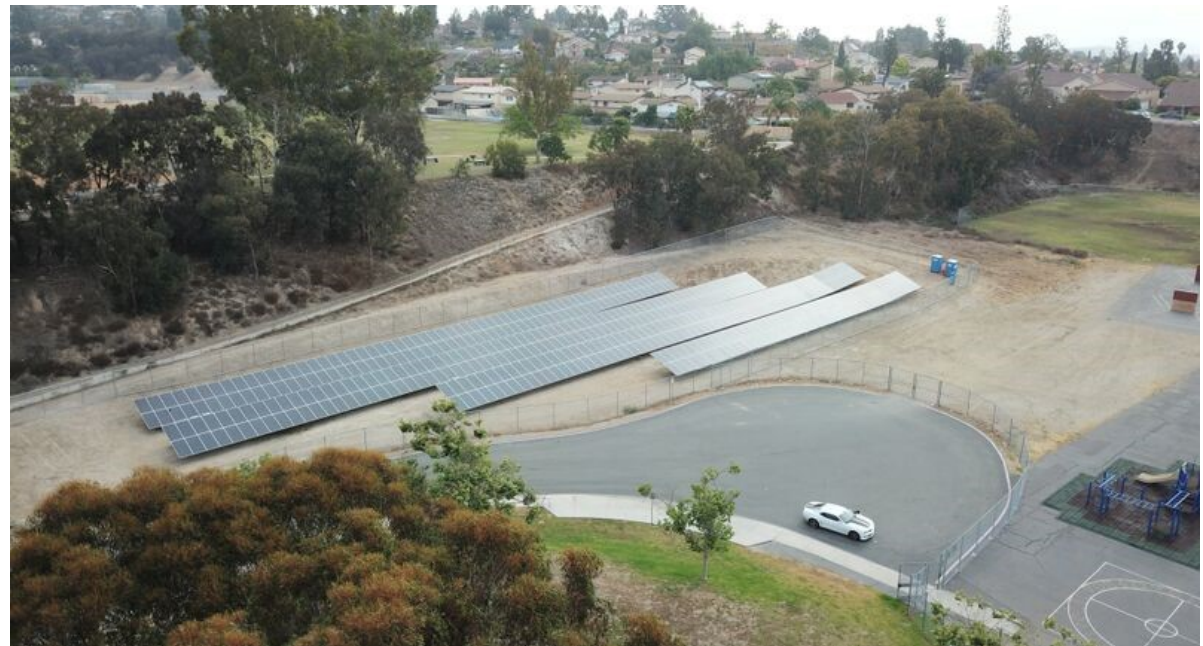
Ground Mount Photovoltaic Solar Panels
