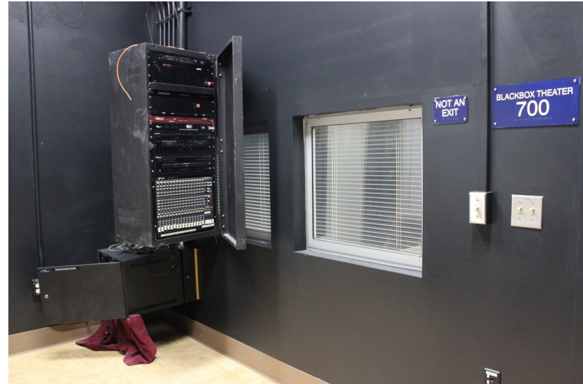
700 building — Black box theater control room
