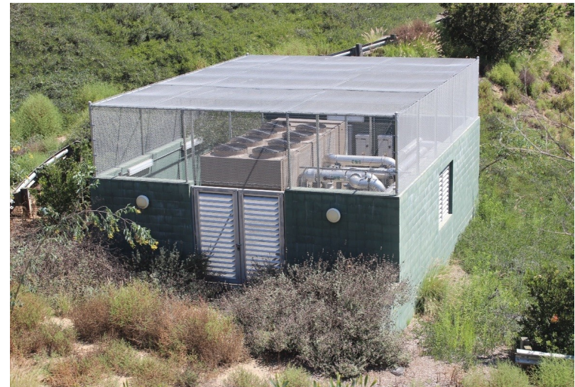
Industrial chiller located in nearby canyon
