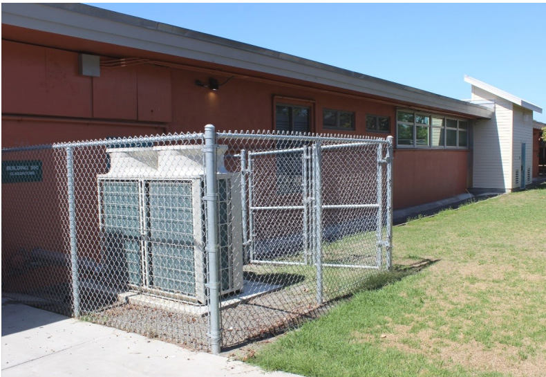
Air conditioning unit and mechanical housing
