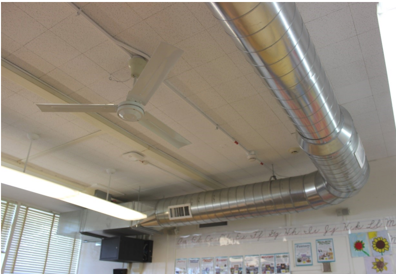
Air conditioning ducts
