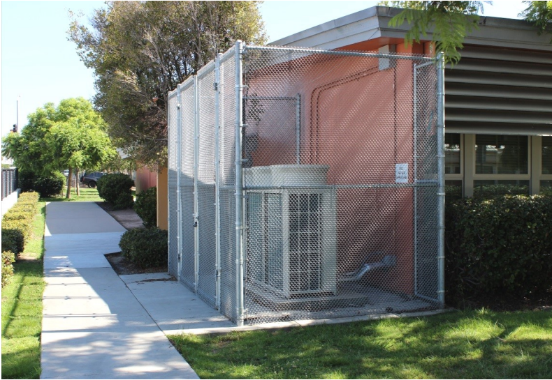
Example of enclosed air conditioning unit
