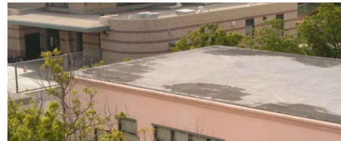
Original roofing area with visible deterioration
