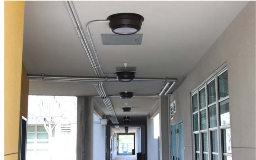
Security lighting in classroom building hallway
