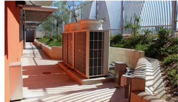
Air conditioning unit
