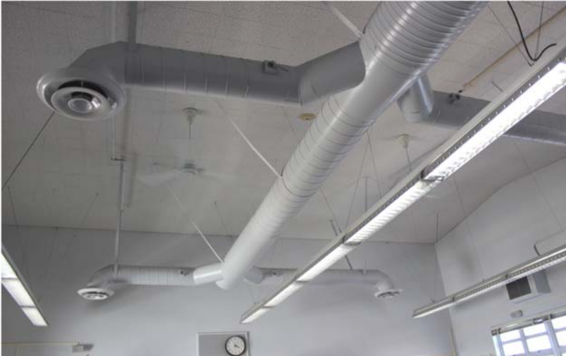
Example of air conditioning ducts found in every classroom
