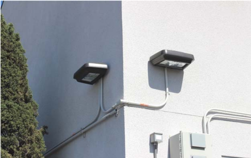
Exterior building security lighting
