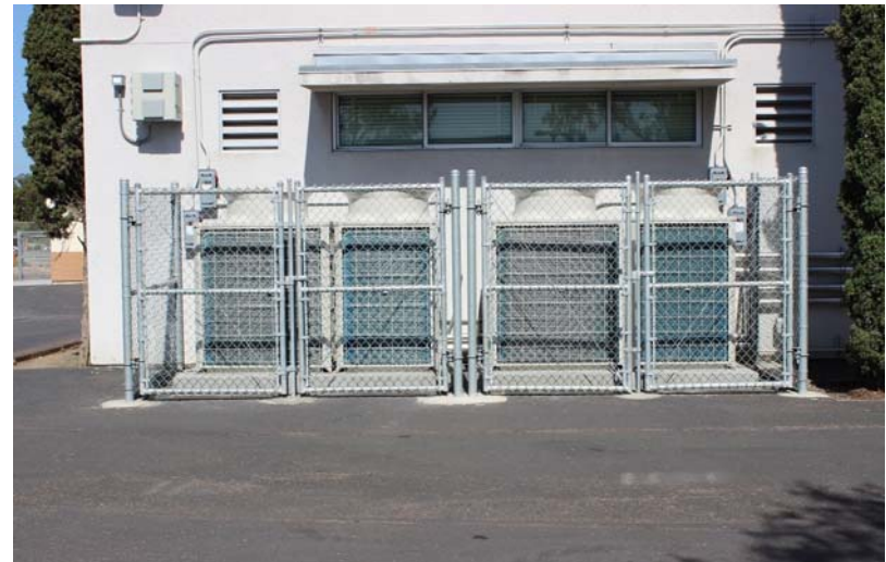
Air conditioning units
