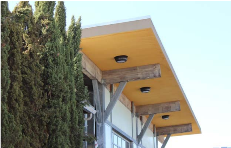
Security lighting on lunch court overhang
