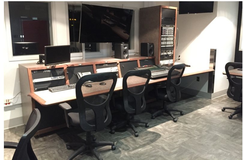
Control room station 2
