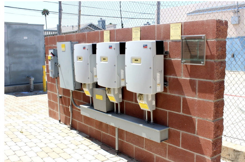
Photovoltaic control panels
