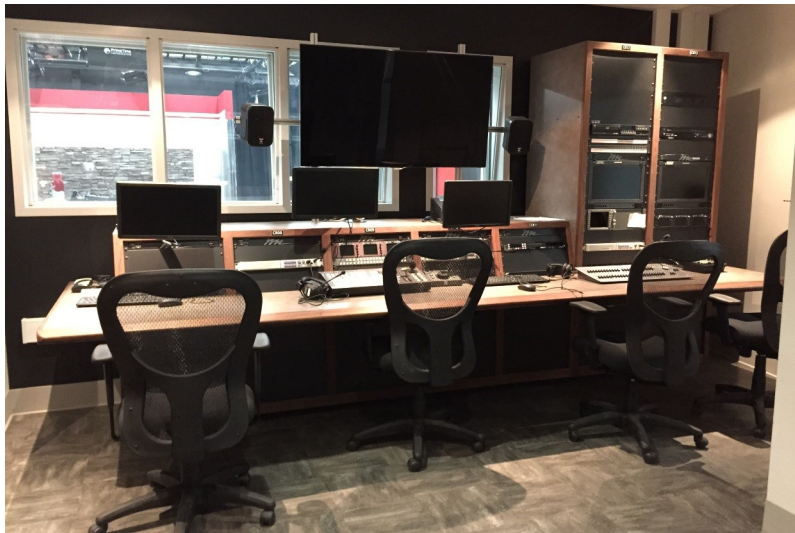
Control room station 1
