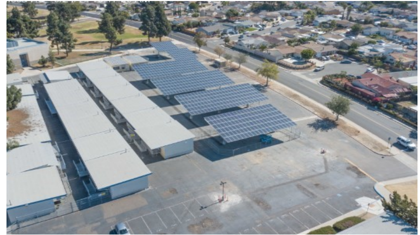
Solar Arrays on the Southeast parking lot
