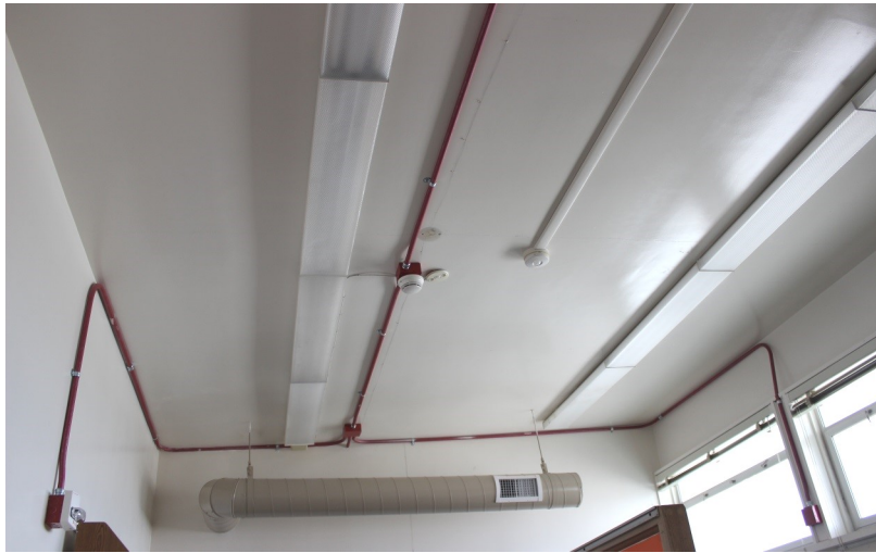
Upgraded fire alarm system and air conditioning added to P.E. areas
