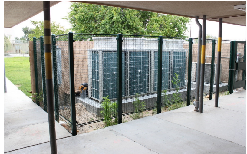
Air conditioning units
