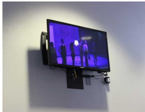
TV in lobby area
