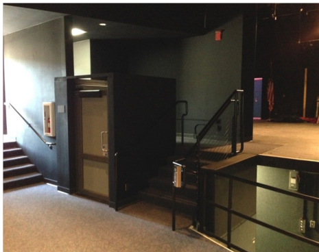
Elevator access to stage
